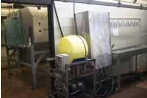
Pump Tank and Spray Chamber
