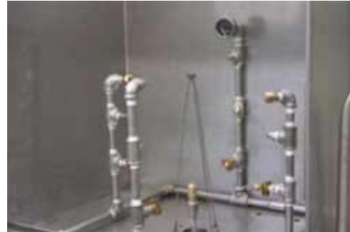
Inside Spray Chamber of Inside/Outside Poultry Washer
